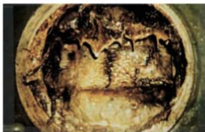
Fig. 4: Blocked fuel line
